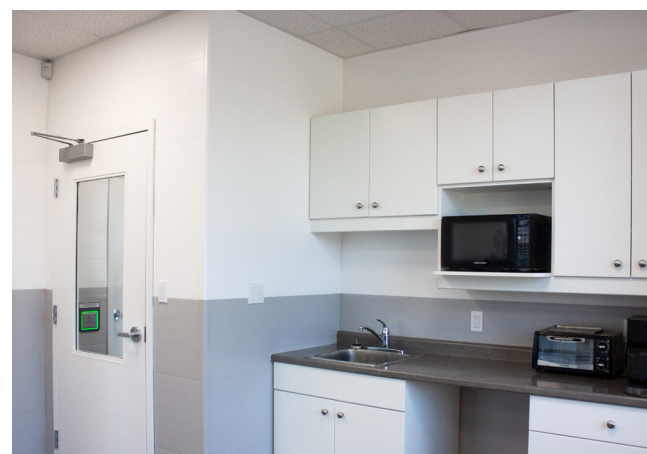
Trusscore Wall&CeilingBoard in Office Cafeteria
