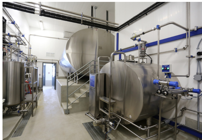
Trusscore Wall&CeilingBoard in Dairy Cleanroom
